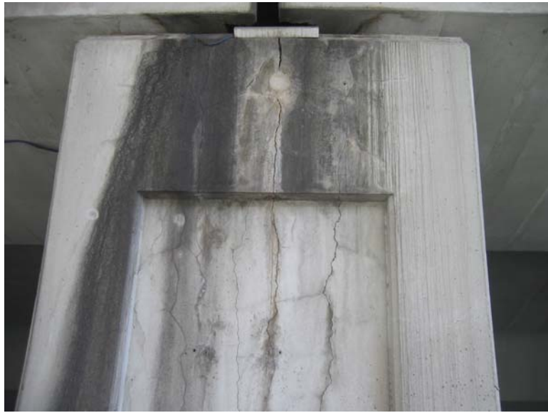
Figure 1.2: ASR and/or DEF Damage in Reinforced Concrete (DD-6)
