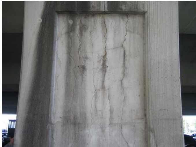
Figure 1.4: DEF Related Damage in DD-6
