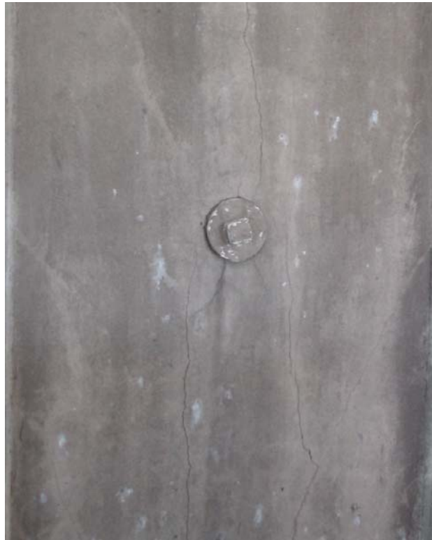
Figure 1.3: ASR and/or DEF Damage in Reinforced Concrete (DD-7)
