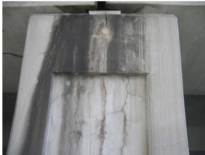
Figure 2.2: Longitudinal Cracking of Spine DD Column
